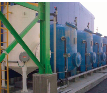
▲ Chemical supply facility that treats the water before the membrane treatment
